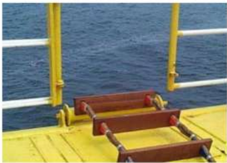
Figure 1: Handholds that terminate above the vessel structure
